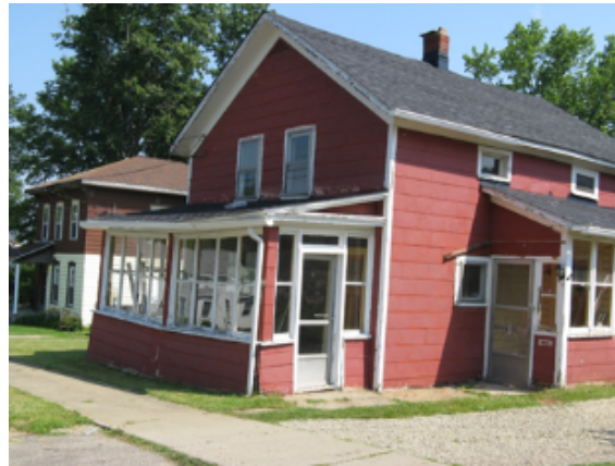
424 S. Center—Vacant, Possible CNI acq. End Use Rehab or Demo w/side lot (70X135)
