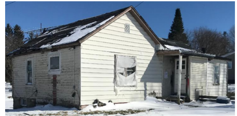
318 Worth—Condemned Unsafe 2 yr. back tax--Possible CNI acq. NW, FNB forgave liens End use Demo—Possible LERTA Build (96X183)
